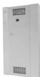
Metering Service Section
