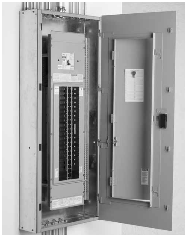
Trim Hanging on Surface Mounted Box
