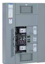
Elevator Control Panelboard
